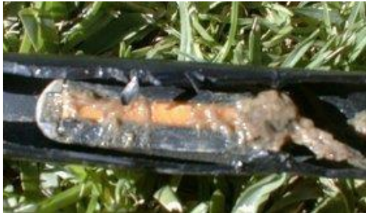
Figure 4 - Biological clogging in a dripper
