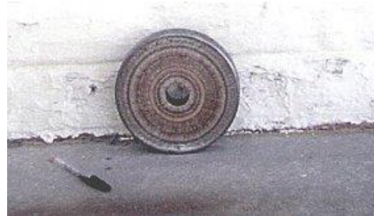
Figure 5 - Pipe internal diameter narrowing
